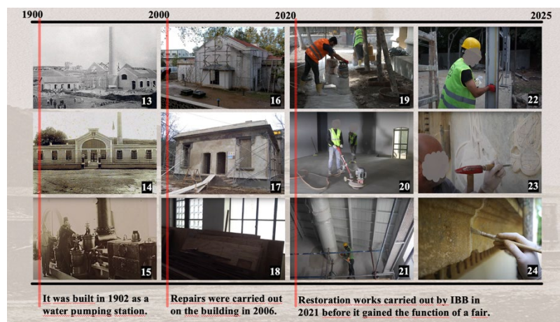
Figure 14 Cendere Art Museum restoration works (TAY Project, n.d. [13,14], Youtube, 2022 [15,18,19,20,21,22,23,24], mimdap, n.d. [16], Rena Construction, 2006 [17], Edited by the authors)
