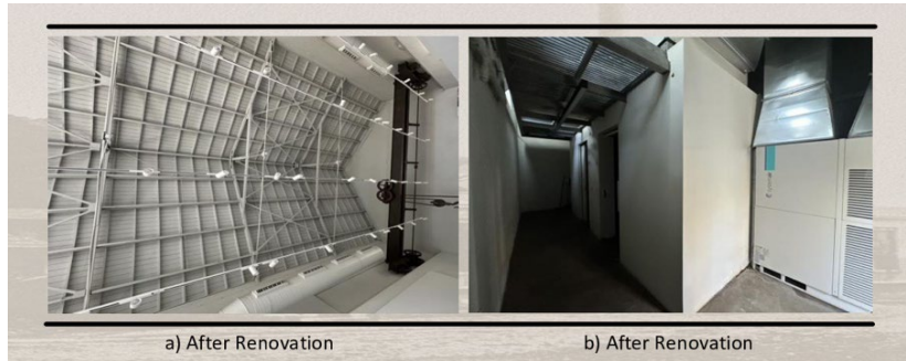
Figure 25 Cendere Art Museum air conditioning system (Photographed by the authors)
